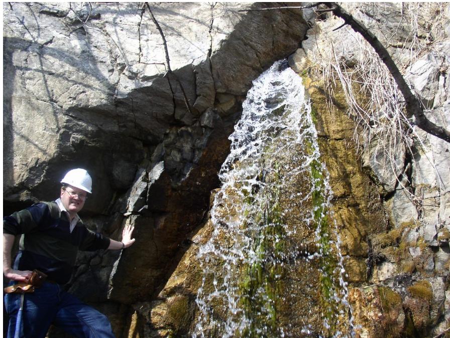
Figure 28. Photo of water-producing discontinuity in quarry wall. Flow is estimated at approximately 200 gpm.
